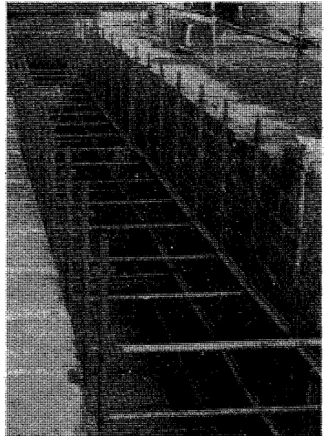
Lock 26E above West Slaithwaite Road bridge, formerly filled in and with a concrete cascade. These have been dug out and the chamber is scaffolded ready to re-point the stonework.
