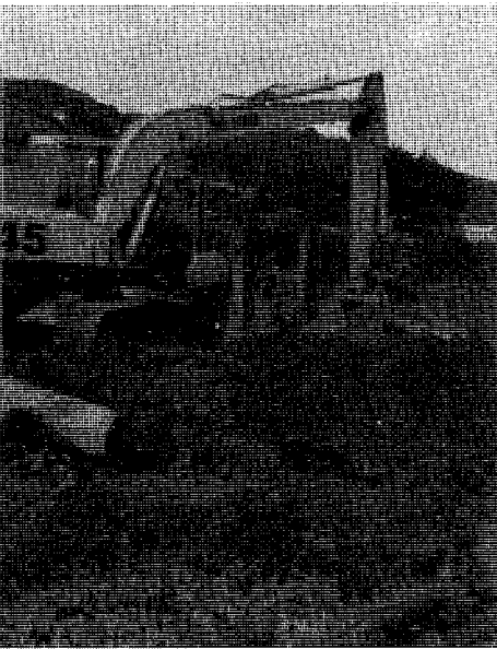
Yorkshire Water Authority workmen re-routing the sewer pipe which crossed the canal below Lock 32E at Sparth.
